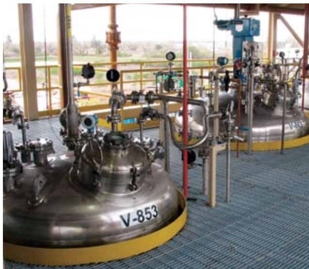
These process vessels are used for handling specialized pharmaceutical intermediates at the Ampac fine chemicals plant in Rancho Cordova.
